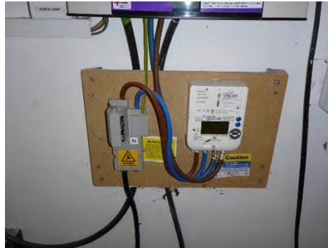
Main fuse & meter
