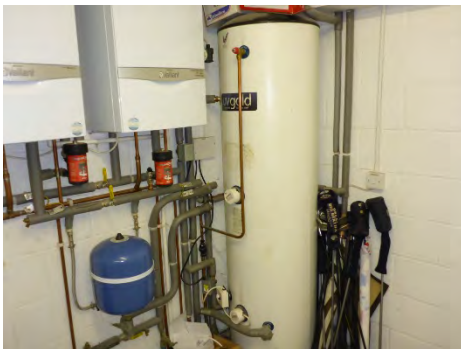
Hot water cylinder
