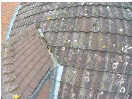
Slipped tile to the right side front dormer
