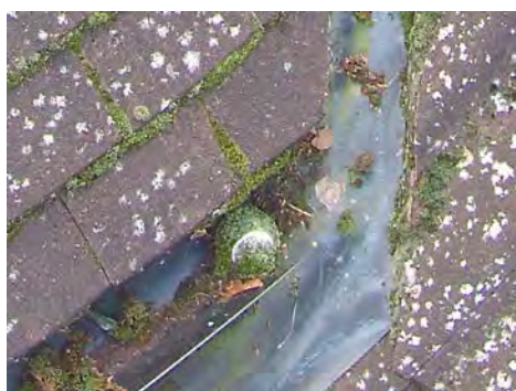
Tennis ball blocking the gutter
