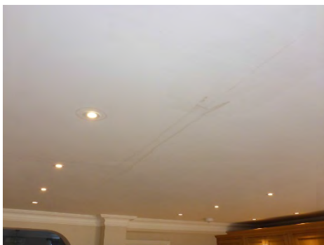
Water stains on ceiling
