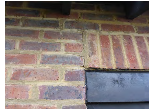
Cracks around window/door heads
