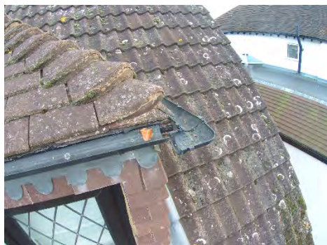
Detached fitting to dormer
