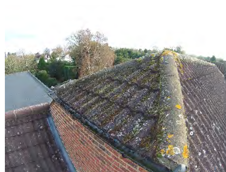
Moss and debris in gutters
