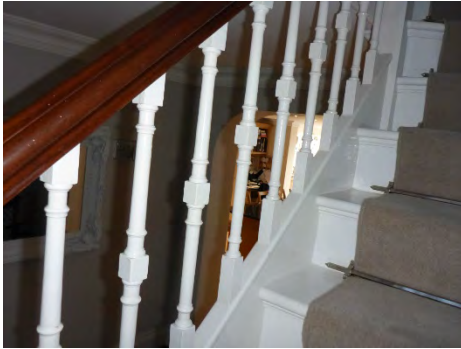
Stair guarding is spaced too wide
