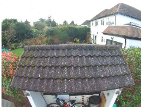
Loose ridge tiles to garden building
