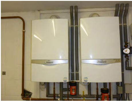
Wall mounted boiler
