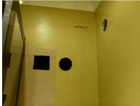
Holes in the wall board
