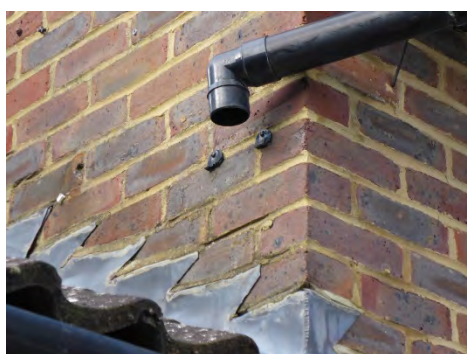
Missing rainwater pipe
