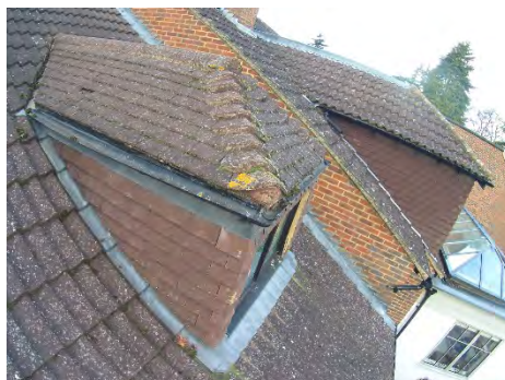
Slipped tile to the right side rear dormer
