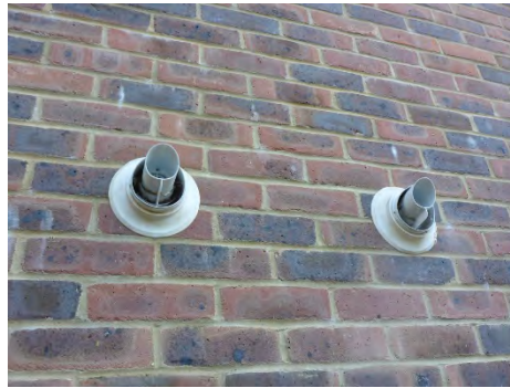
Fan assisted flue
