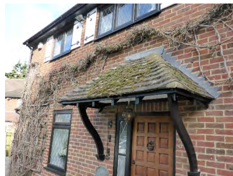
No gutters to the porch
