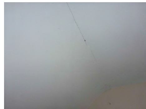
Skeiling cracks inside the cupboard
