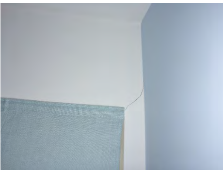
Wall crack above window
