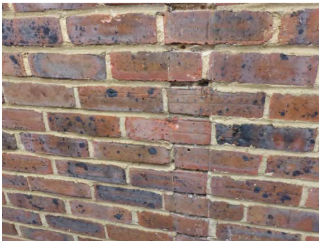
Loose and missing pointing to the side
