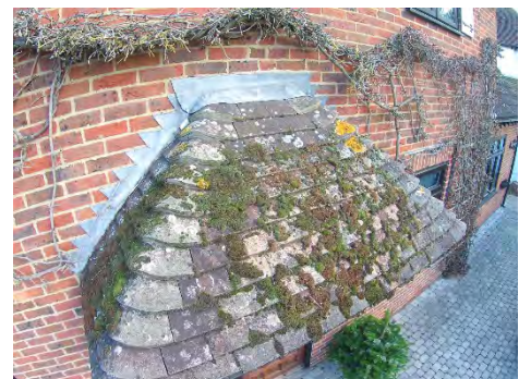
Moss on porch roof tiles
