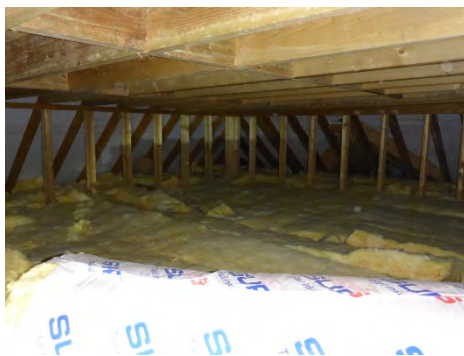
Extension roof has no central bracing
