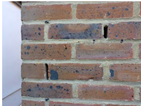
Holes in the rear wall
