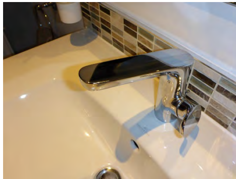
Tap to wash hand basin is loose
