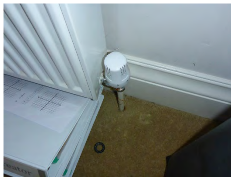
TRV's fitted to radiators
